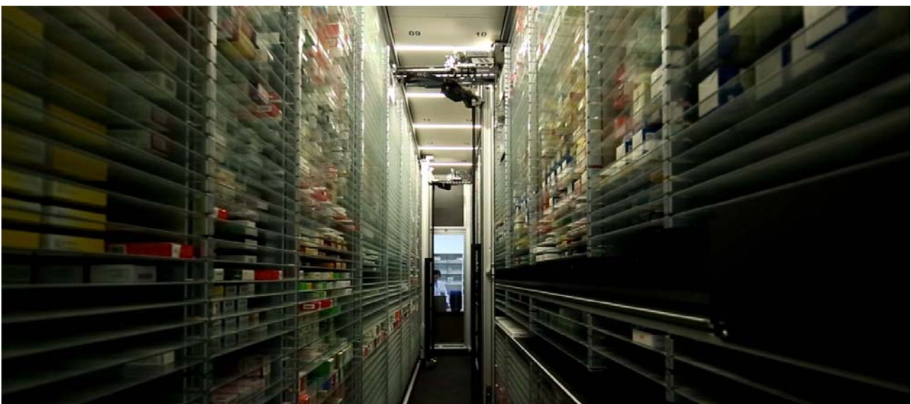
Example of good practices: storage automated pharmaceutical storage room - Maternal and Child Hospital, Shenzhen, China
